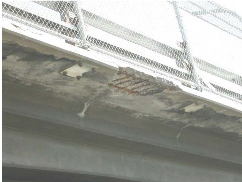
Fig. B1.5.1 Spalling on the bottom of the pedestrian lane
