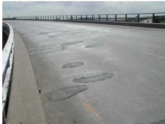
Fig. C.1.14. The corrosion damage before the repair of the bridge deck
