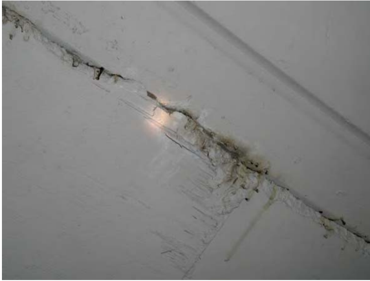
Fig. B1.4.7 Bottom deck view - seepage of water around the construction joint
