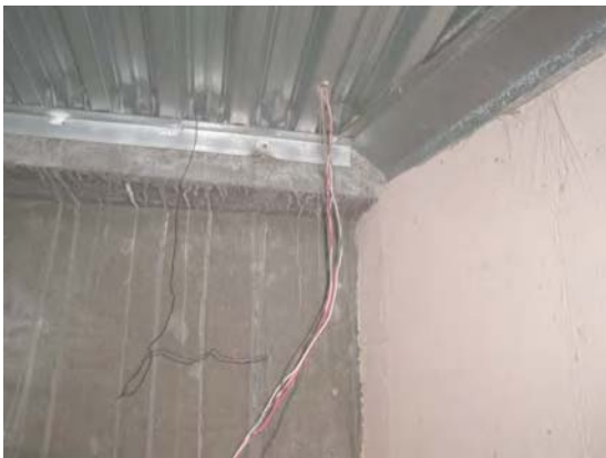
Fig. C.5.4 The wires of the corrosion monitoring system
