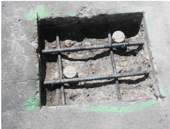
Fig. 3.3 The Galvashield cathodic protection system installed in SH 85 SB in Greeley, Colorado.
