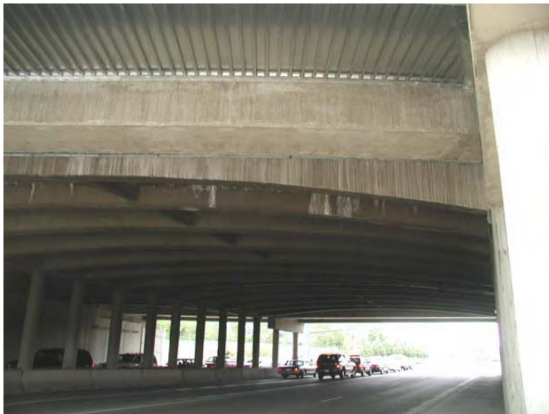
Fig. B1.2.8 Leakage on the bottom deck - on the construction joint
