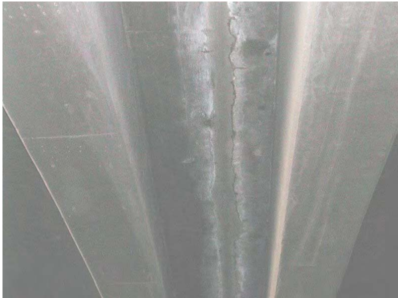
Fig. B1.5.4 Severe cracking
