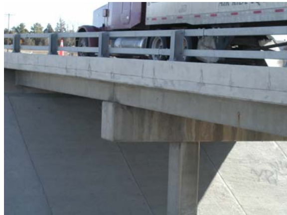
Fig. 1.2 Corrosion damage on pier caps
