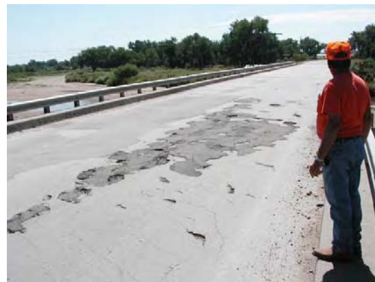
Fig. C.2.8 The severe corrosion damage before the repair of the bridge deck
