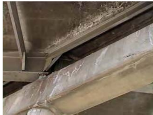
Fig C.1.9 Salt deposited on the pier cap and connection between girder and deck
