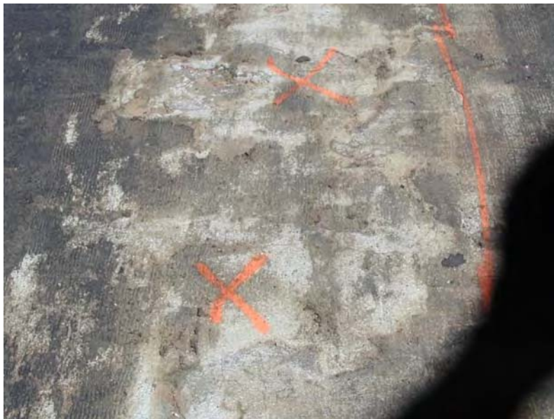
Fig. B1.4.2 A marked area of delamination on the deck – tested using hammer sound
