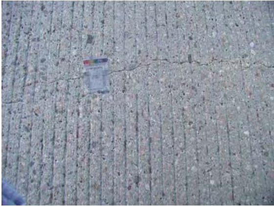
Fig. C.6.8 Transverse crack with width varying from 0.016-0.030 in
