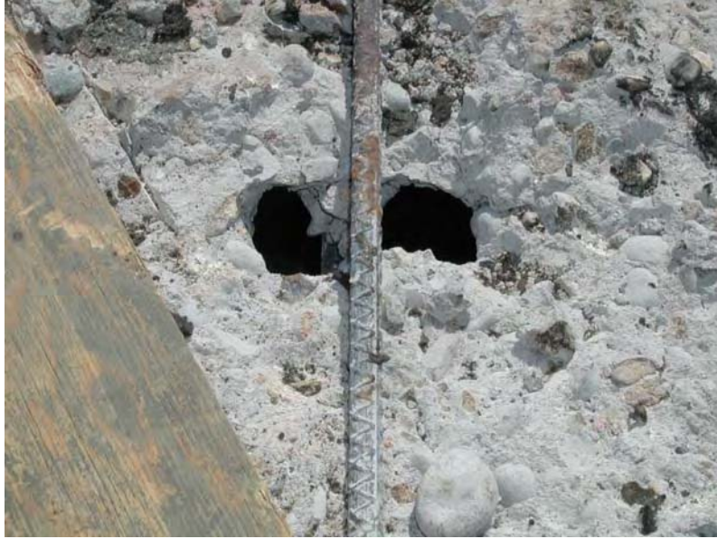
Fig. B1.4.3 Slab floor is heavily damaged (a big hole in the deck)
