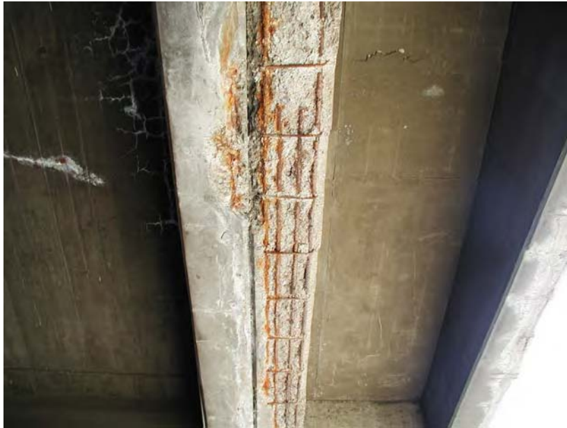
Fig. B1.7.3 Heavy spalling and corrosion on one of the girders
