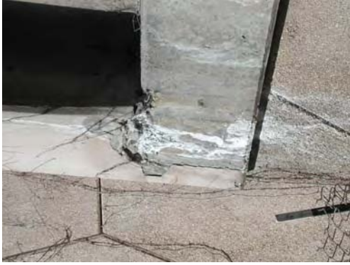
Fig. C.9.5 The flow of deicing salt near construction joint
