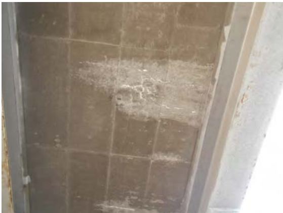
Fig C.1.4 Efflorescence on the bottom of the bridge deck
