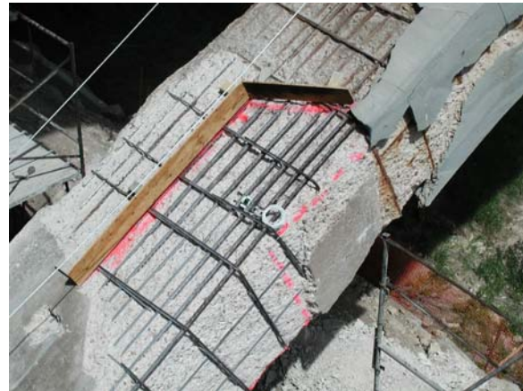
Fig. 3.2 Repair corrosion damage on the arch
