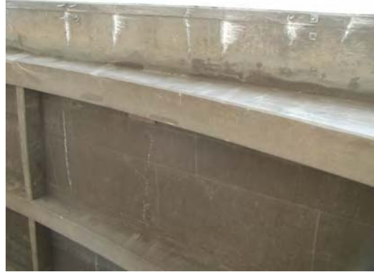
Fig. C.8.9 Efflorescence on the shoulder
