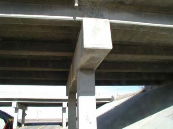
Fig. C.6.10 Cracks on a pier cap
