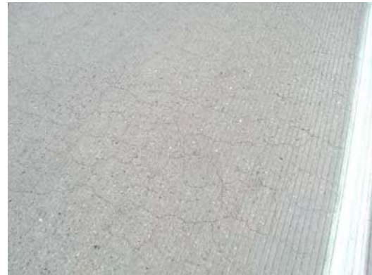
Fig. C.7.7 Cracks on the deck slab
