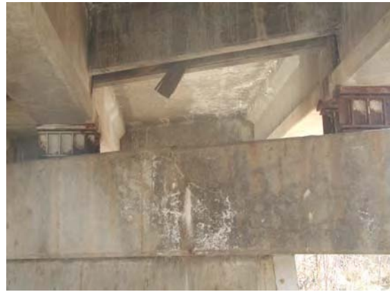
Fig. C.2.6 Efflorescence on the bottom and pier cap
