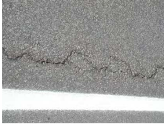
Fig. C.8.5 A longitudinal crack on the asphalt overlay
