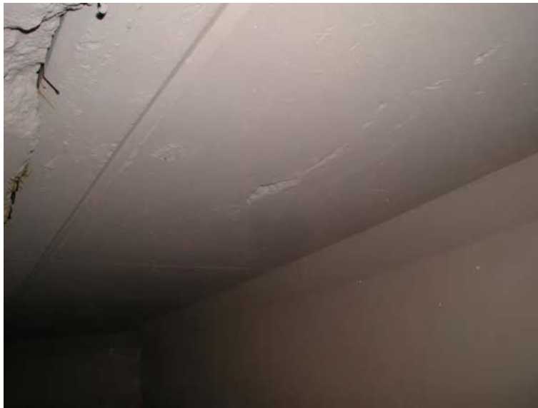
Fig. B1.4.8 A major cracks on the bottom deck
