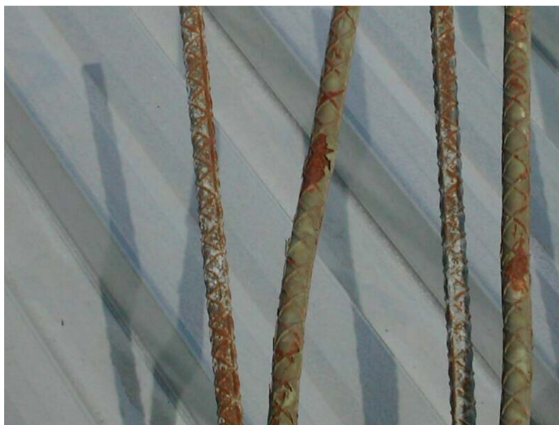
Fig. B1.1.2 Corrosion of epoxy-coated rebars
