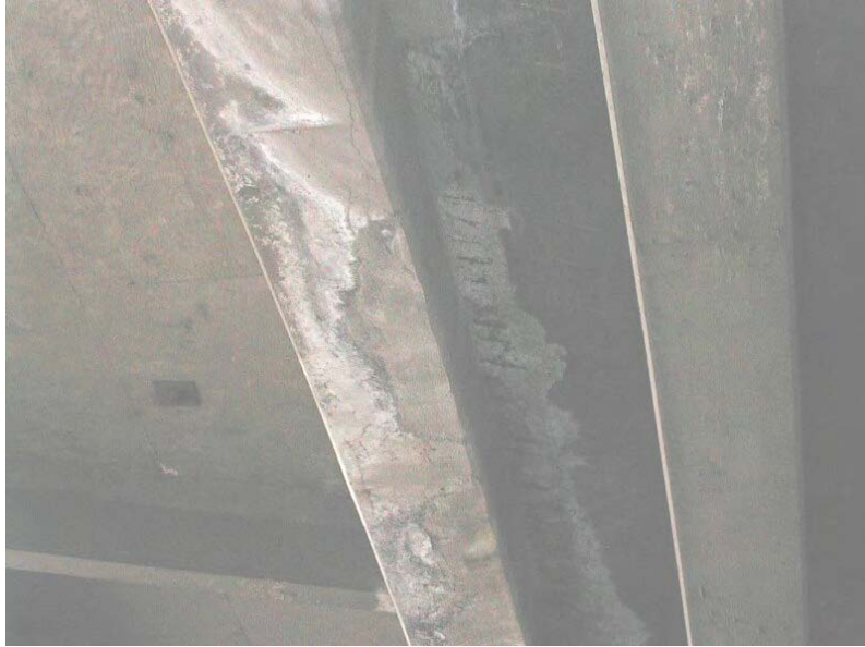
Fig. B1.5.3 Efflorescence on the main beam (girder)
