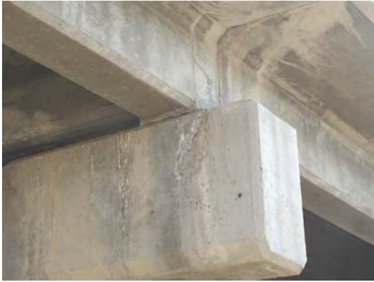
Fig. C.7.8 The concrete spalling with efflorescence on one of the pier caps
