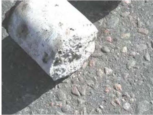
Fig. C.9.7 A concrete core extracted from the shoulder lane
