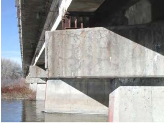
Fig. C.2.3 Cracking and spalling on the pier cap
