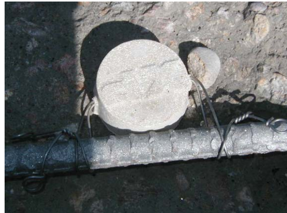
Fig. 3.4 A close view of the Galvashield cathodic protection system.
