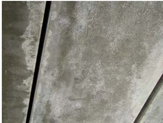
Fig. C.3.7 Efflorescences at the bottom of bridge decks
