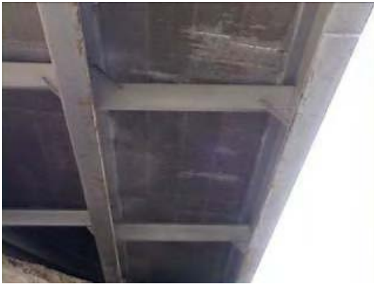
Fig C.1.8 Efflorescence on the bottom of bridge deck
