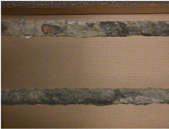
Fig. 1.1 Corroded steel bars on one of the bridges in I-70
