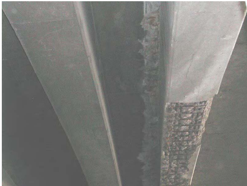
Fig. B1.5.6 Severe spalling and corrosion on the main beam (girder)
