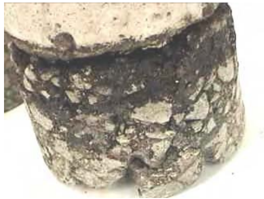
Fig. C.8.14 Damaged asphalt membrane overlay (cracked area - driving lane)
