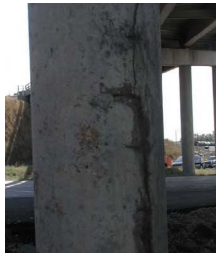
Fig C.1.7a Spalling on a pier before the placement of asphalt overlay on the deck
