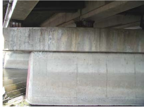
Fig. C.2.4 Cracking on the pier cap
