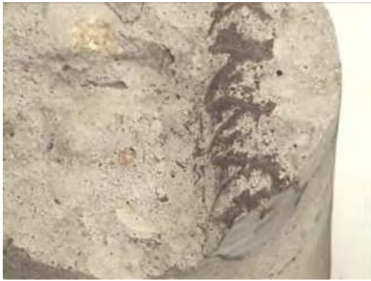
Fig. C.8.13 A corroded steel bar (in the shoulder lane)
