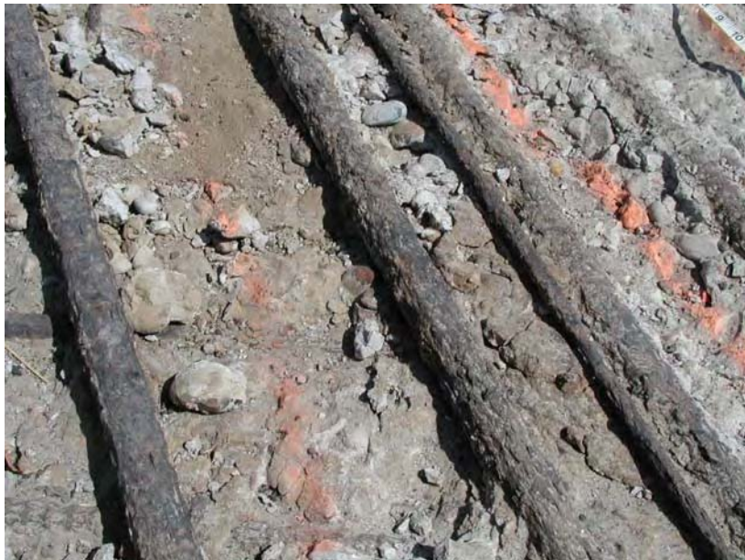
Fig. B1.4.4 Severe corrosion of main reinforcement steels
