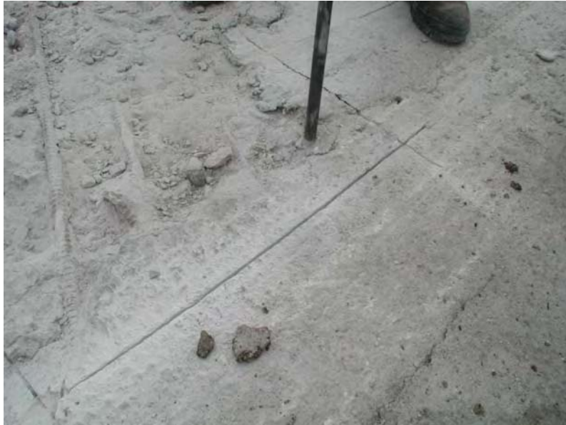
Fig. B1.2.3 Delamination test – heavy delamination was encountered
