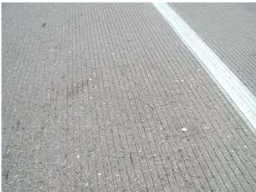
Fig. C.7.6 Cracks on the deck slab
