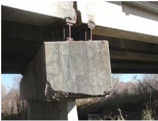
Fig. C.2.5 Spalling on the pier cap
