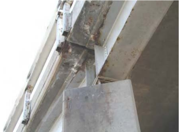
Fig C.1.5 Efflorescence and corrosion damage on the lower elevation (slope) of the bridge
