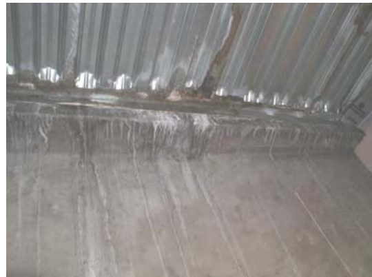
Fig. C.5.7 Efflorescence – seepage of salt on the bottom of bridge deck
