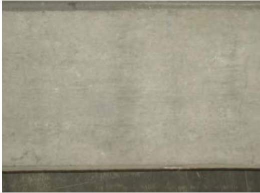
Fig. C.8.8 Cracks on the transverse girder
