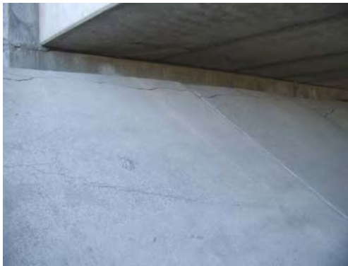
Fig. C.3.10 Cracks around the bridge abutment
