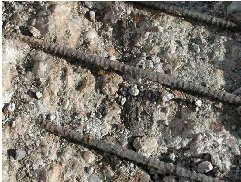
Fig. B1.2.4 Corroded steel on the concrete deck
