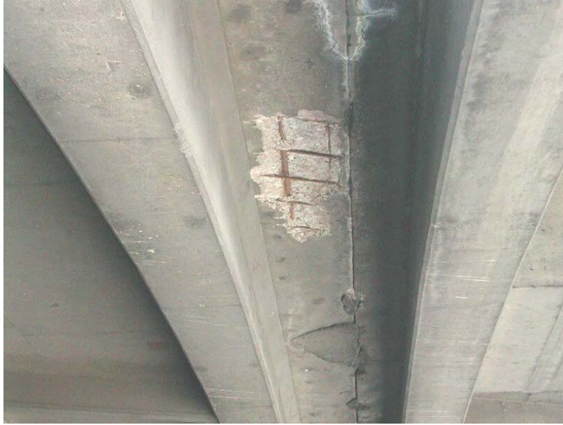
Fig. B1.5.7 Severe spalling on the bottom deck
