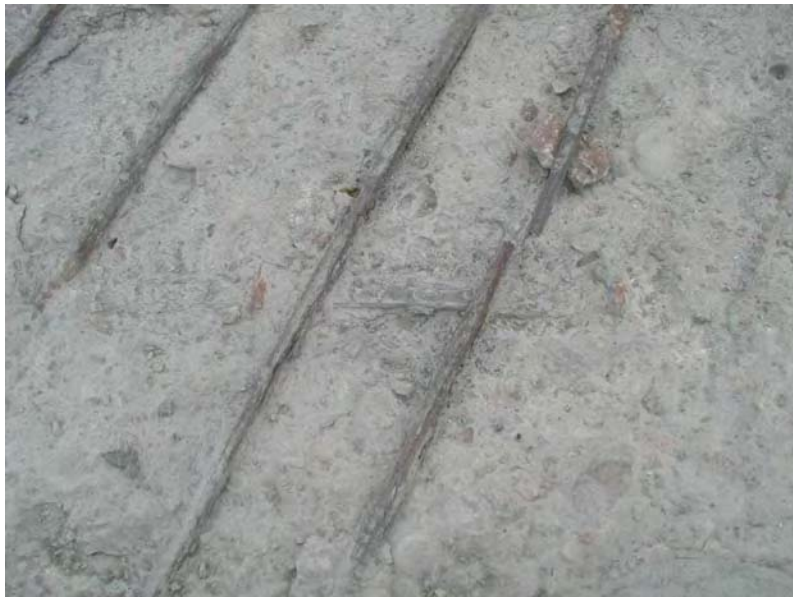
Fig. B1.2.6 Severe corrosion of steel bars
