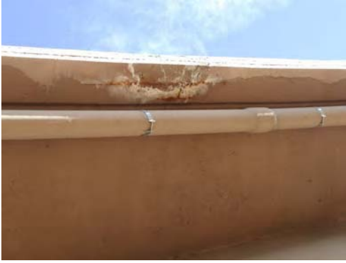
Fig. C.9.4 Efflorescence on the overhang structure
