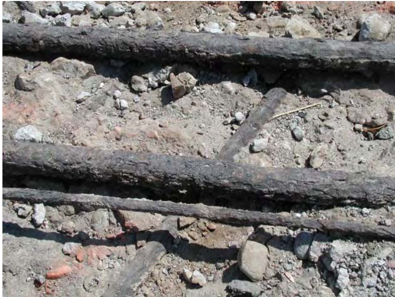
Fig. B1.4.5 Severe corrosion of main reinforcement steels
