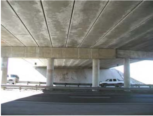
Fig. C.3.8 Efflorescence on the bottom deck
