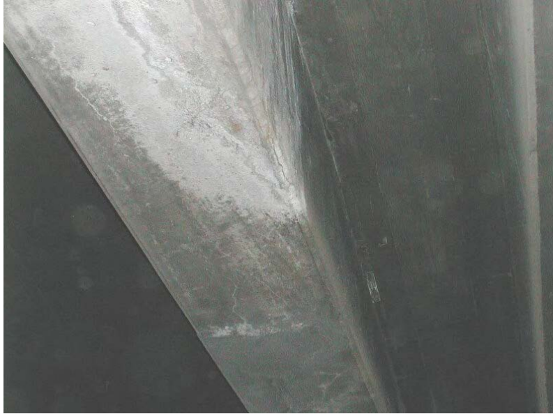
Fig. B1.5.5 efflorescence on the main beam (girder)
