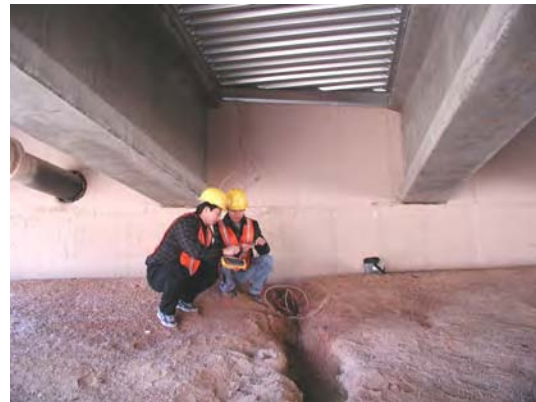
Fig. C.5.5 Corrosion potential measurement – to detect corrosion activity
