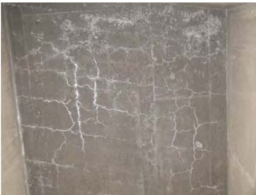
Fig. C.8.6 Efflorescence with crack pattern on the bottom of the slab (I)
