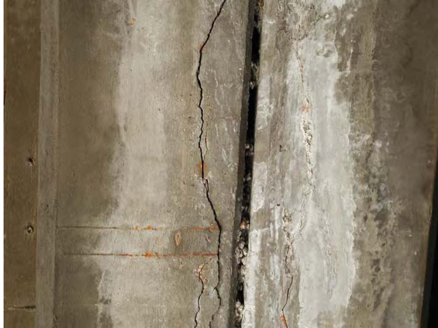
Fig. B1.7.5 Severe cracking in one of the girders near efflorescence areas
