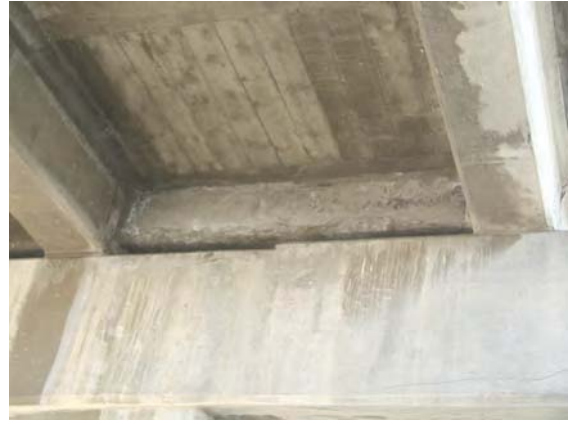
Fig. C.6.9 Severe spalling on the sub-beam
