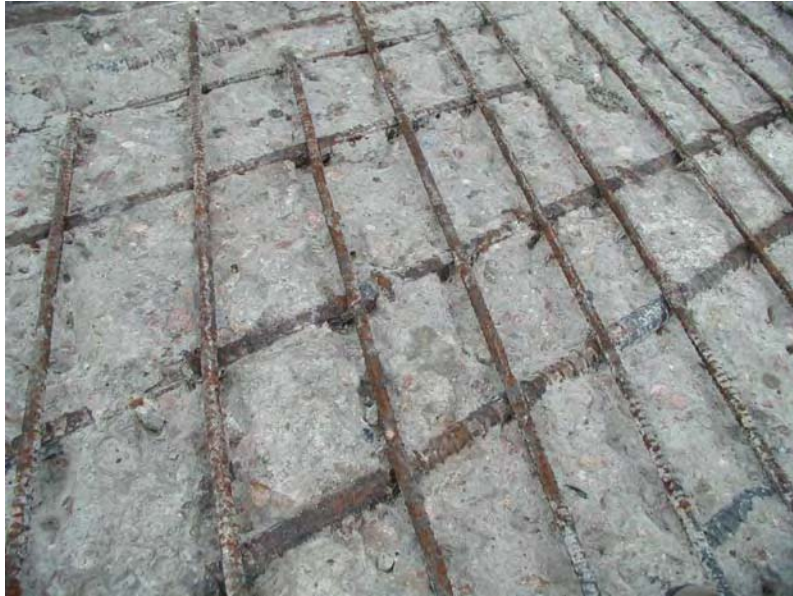
Fig. B1.2.7 Large area of corroded steel bars in the deck
