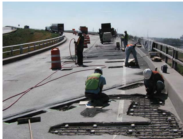
Fig. C.1.15. The Galvashield corrosion protection system installed on some parts of the bridge deck
