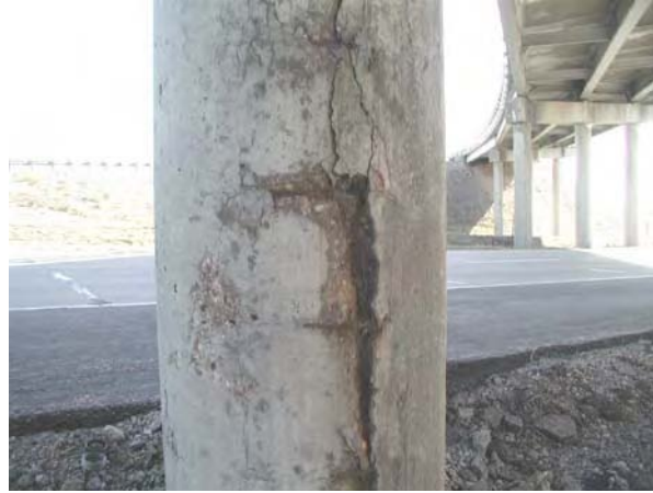
Fig C.1.7b Severe spalling on the same pier after the placement of asphalt overlay on the deck
