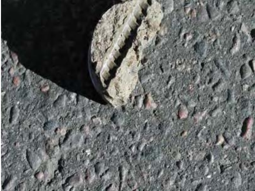
Fig. C.9.8 No signs of corrosion rust/deposit found on the concrete cover on an epoxy-coated rebar
