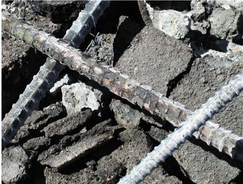
Fig. B1.7.7 Corrosion of steel bars
