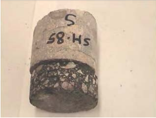
Fig. C.1.12 Cracking in the core – shoulder lane
