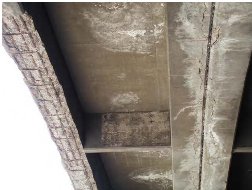
Fig. B1.7.4 Corrosion of steel and spalling of concrete in another girder
