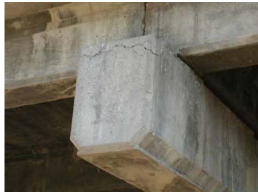
Fig. C.7.5 Cracks on one of the pier caps
