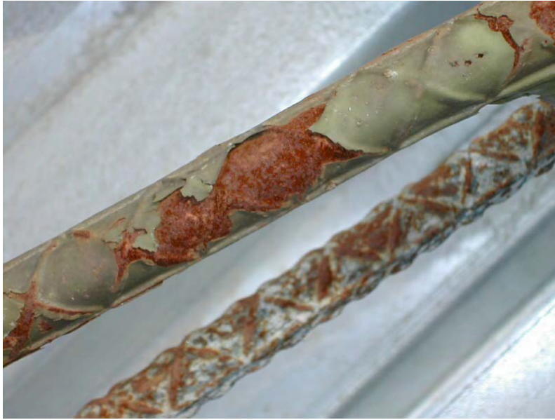
Fig. B1.1.3 Close view of corrosion of epoxy-coated rebars
