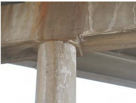
Fig C.1.6 Cracks on the pier and salt deposited on the pier cap
