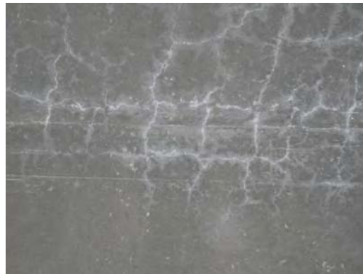
Fig. C.8.7 Efflorescence with crack pattern on the bottom of the slab (II)
