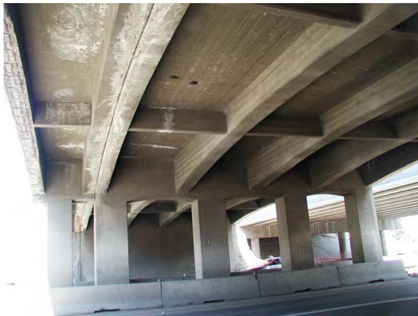
Fig. B1.7.2 Heavy spalling and efflorescence on the bottom of deck
